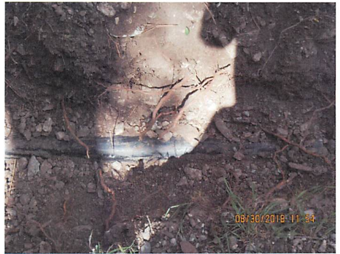
Photo 2: Exposed Building Sewer Line for 4721 Aspen Ave
