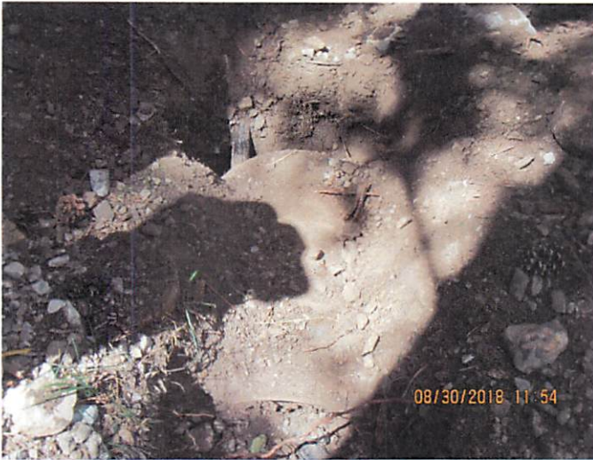
Photo 1: Unpermitted ISDS to Service the Laundry Room
