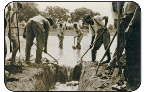
Workers practicing "vector control" in 1920 by digging a drainage ditch, in order to help disperse standing water that was acting as a popular breeding ground for a population of Anopheles mosquitoes, a well known vector for the parasitic disease, malaria. Photo Credit: CDC Public Health Image Library
