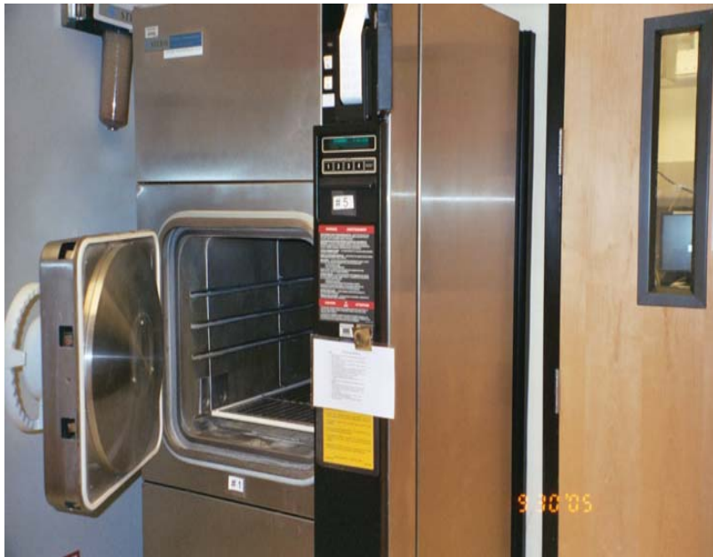
Pass through decontamination autoclave
